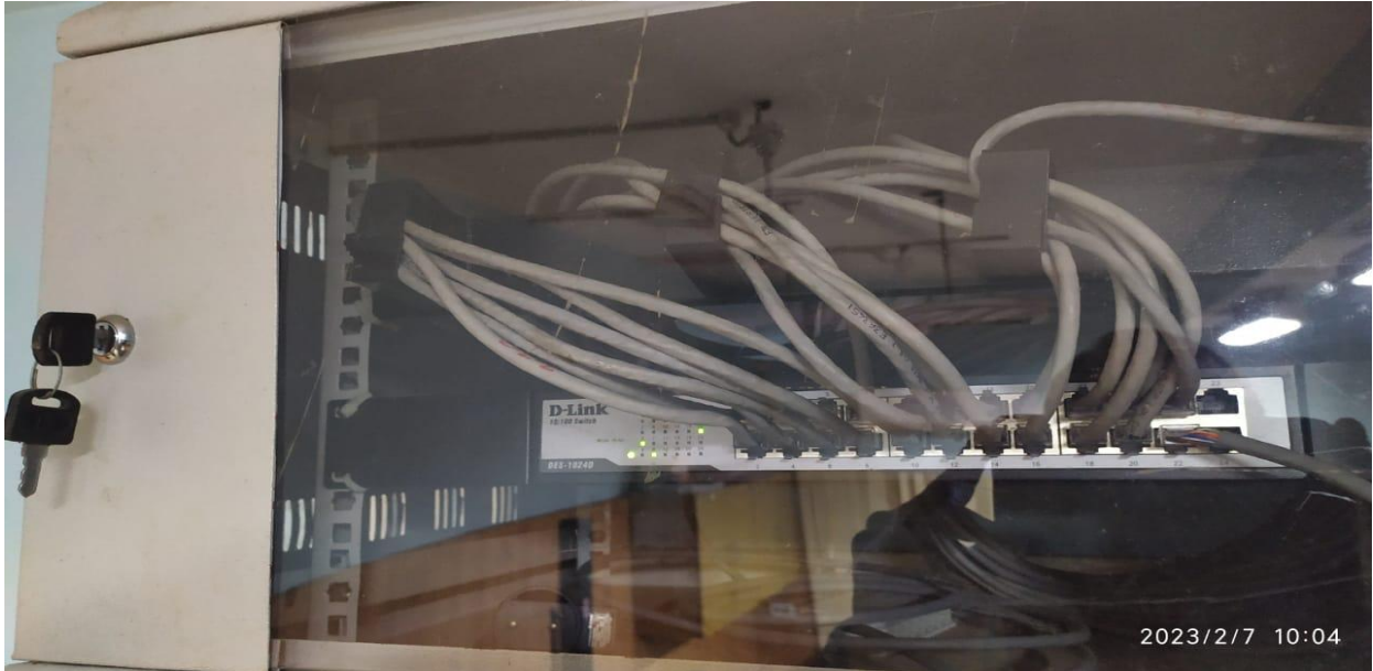
ETHERNET SWITCH IN CABINET
