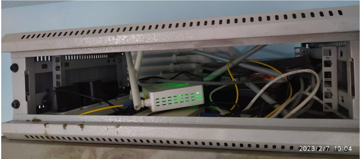
ROUTER IN CABINET
